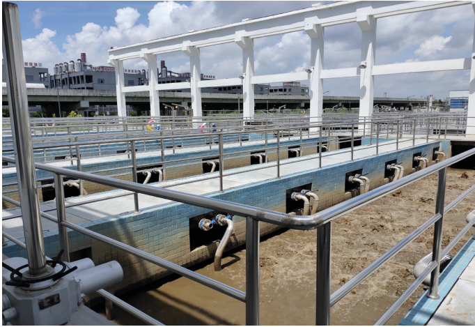
Municipal MBR in Guangdong, China Capacity, 30,000 m 3 /d
