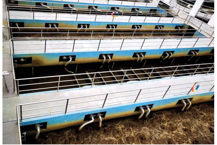
Municipal MBR in Guangdong, China Capacity, 50,000 m 3 /d
